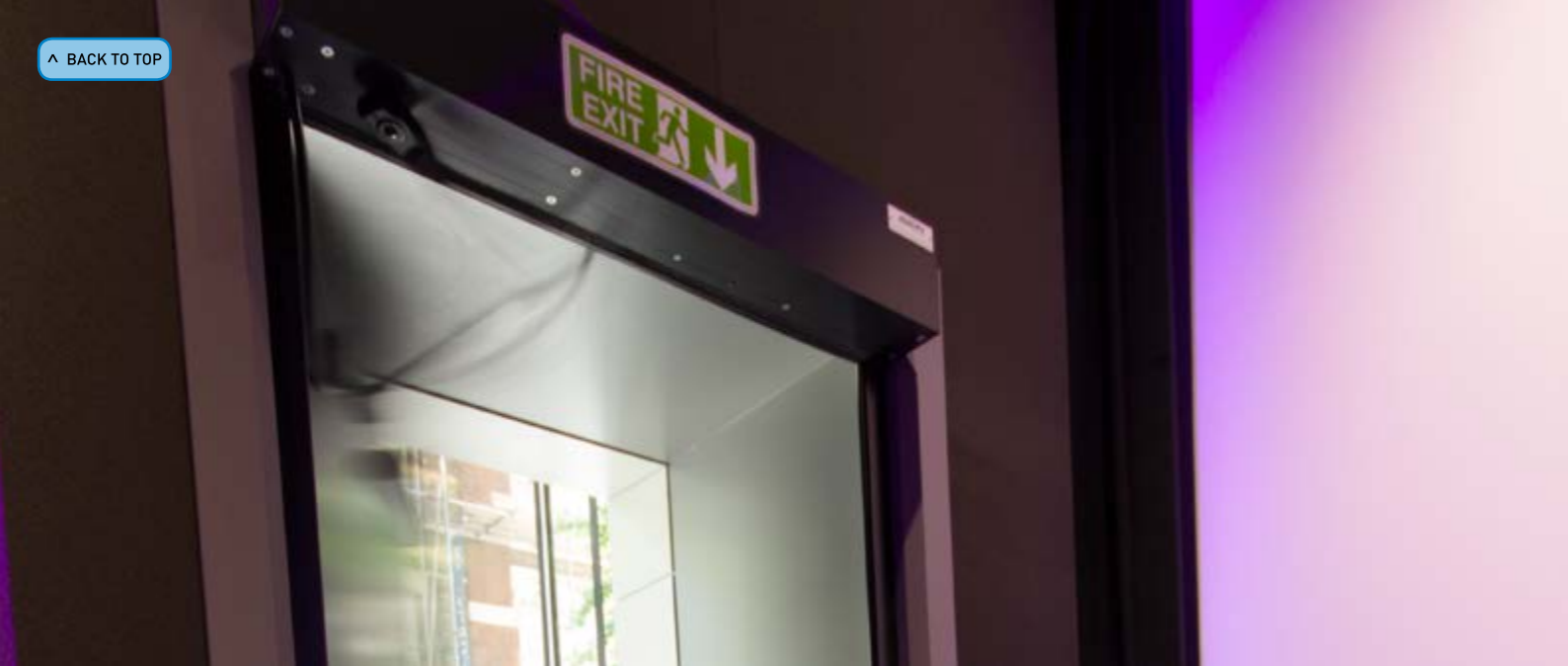
FD20 Automated Operators at NBC Universal Theatre, London, UK
