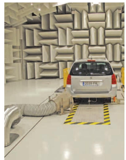
Exhaust gas extraction installation in vehicle hemi-anechoic chamber
