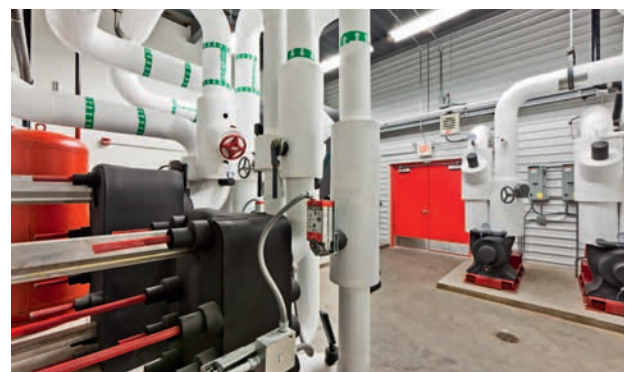
Plant room for turnkey acoustic testing facility
