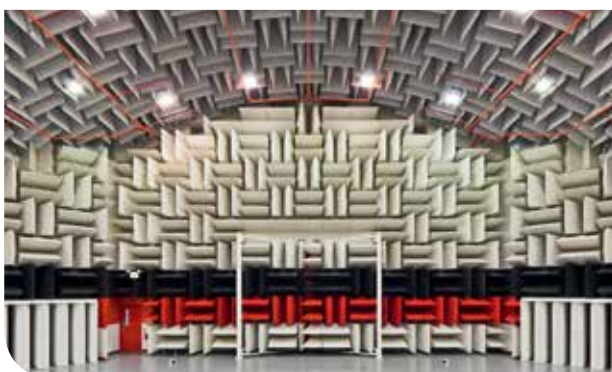
Hemi-anechoic room highlighting IAC's chosen lighting system alongside the client's preferred fire suppression system
