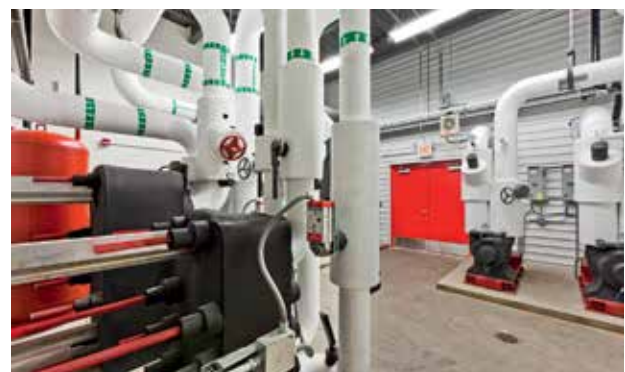
Plant room for turnkey acoustic testing facility
